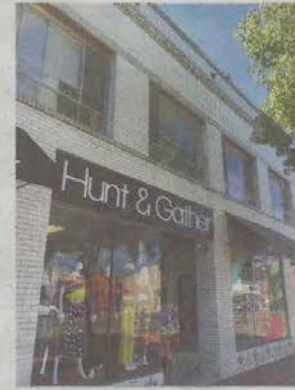
The mosaic tile trim below the display windows of Hunt and Gather at 2871 University Ave. and A7D Creative Group at 2867 University Ave. was recently restored.
